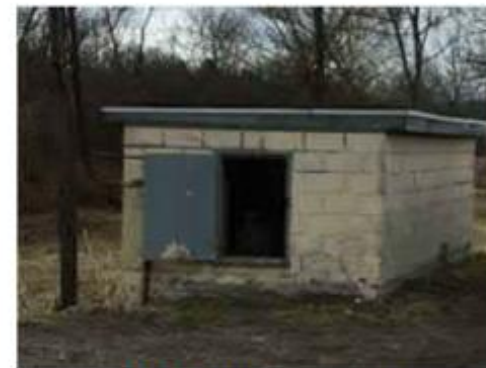
Well House No. 2
