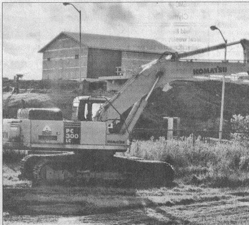
The Village of Sherman Waste Water Treatment Plant Improvement project has been proceeding on schedule with only a few change orders.
